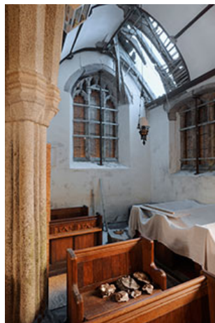
Damage to the roof of the church © Richard Downer
